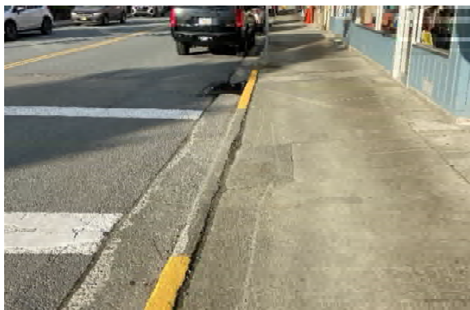
Photo 4 - Pedestrian Ramp lacking detectable warning mat and flat landing
