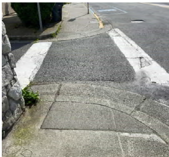
Photo 5 – Pedestrian Curb Ramp lacking detectable warning mat
